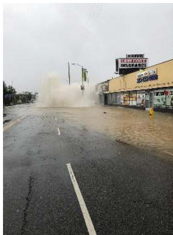
Figure 4.1.8: Pipe Rupture Image Source by Los Angeles Fire Department is licensed under CC BY-ND 2.0
